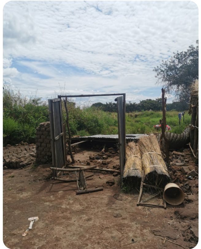
Figure 10: market stall in Alel Thoy damaged by flooding in 2022.
